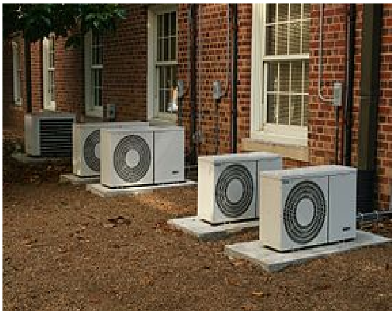
Figure 71:- Air conditioning units outside a building
