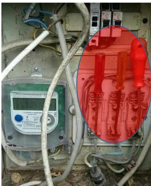
Figure 70: Dangerous fuse 'replacement'
