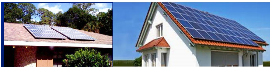
Figure 13 : Roof mounted solar module
