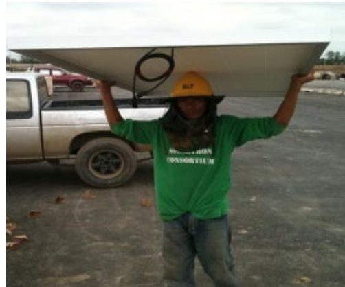
Figure 103: Wrong way to carry a module
