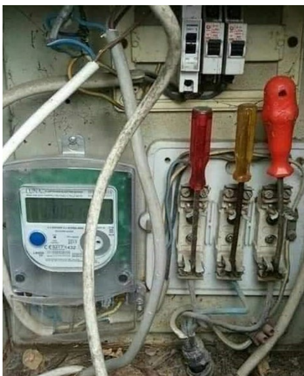
Figure 27: Wrong fuse 'replacement'
