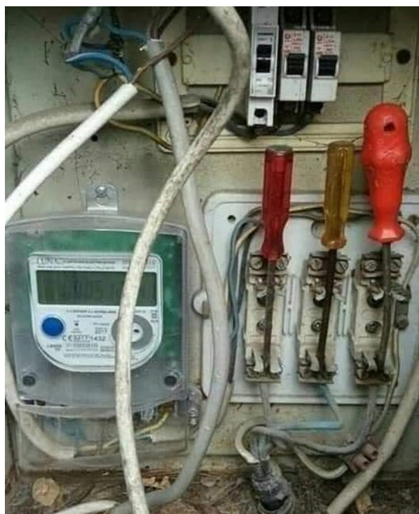
Figure 34: Wrong fuse 'replacement'
